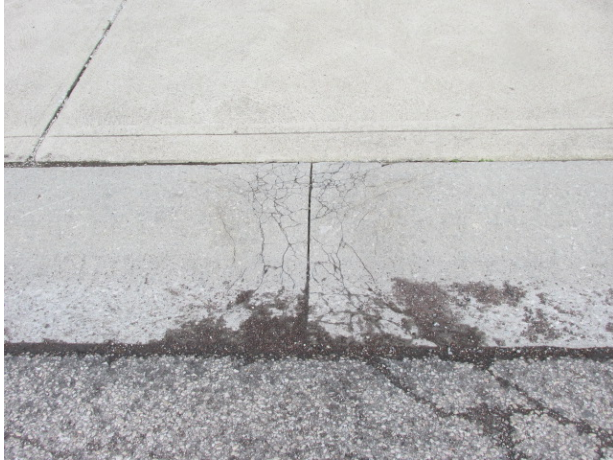
Cracks and deterioration at curb and gutter
