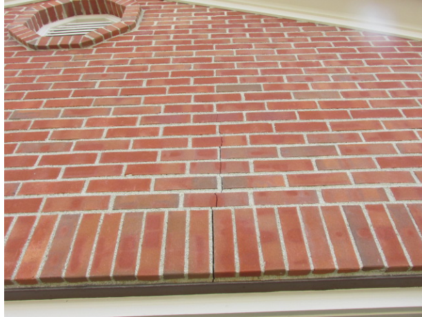
Crack at masonry above garage
