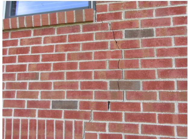
Step crack at masonry
