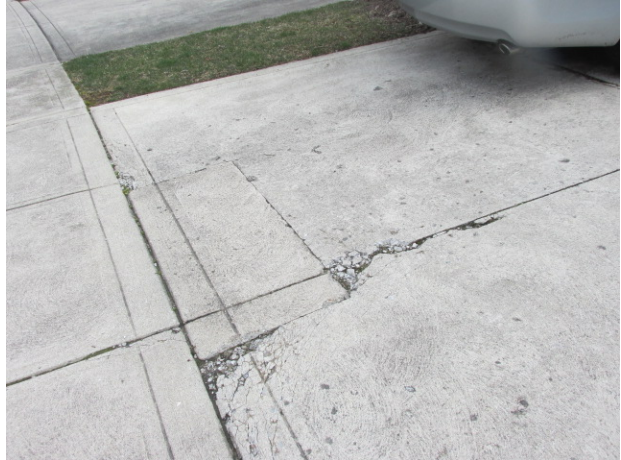
Cracks and deterioration at driveway
