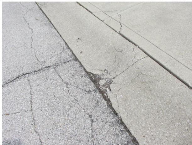
Cracks and deterioration at curb and gutter
