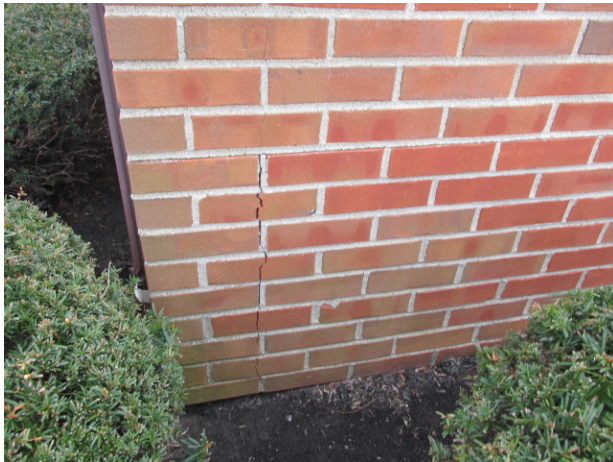
Crack at masonry
