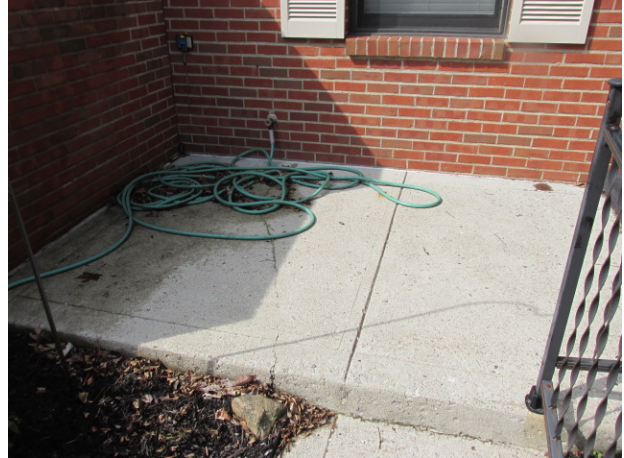
Crack at concrete stoop
