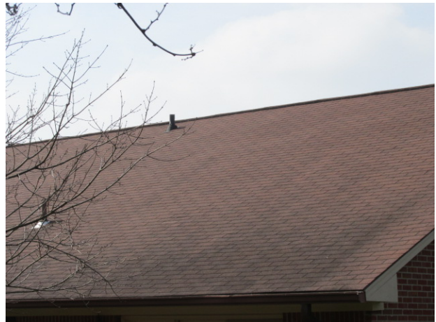
Discoloration at asphalt shingle roof
