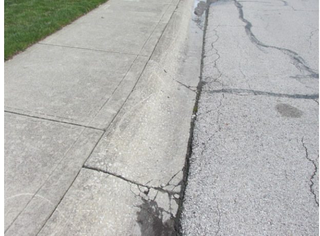
Cracks and deterioration at curb and gutter
