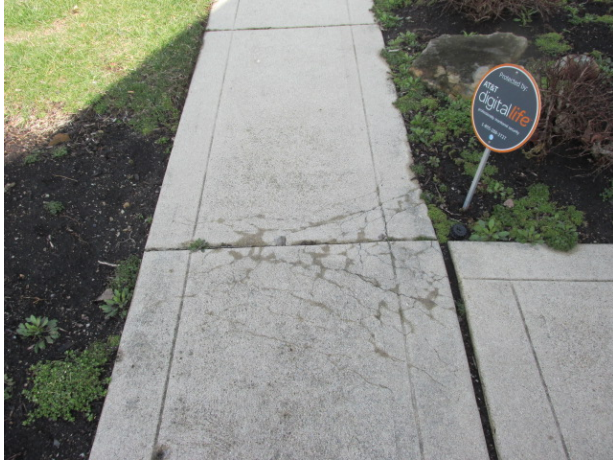
Cracks at sidewalk
