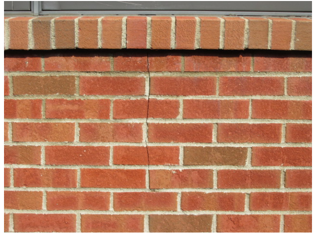
Crack at masonry
