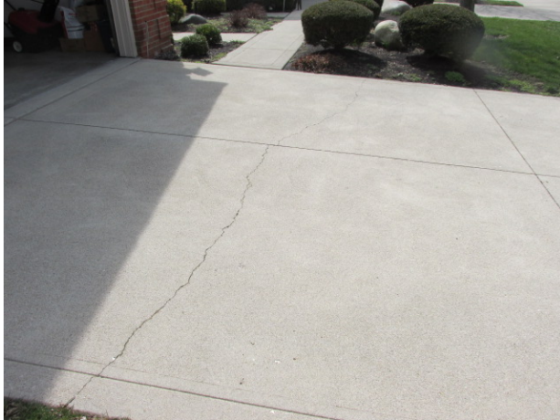
Crack at driveway
