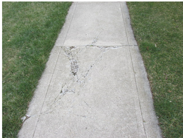
Cracks at deterioration at concrete sidewalk
