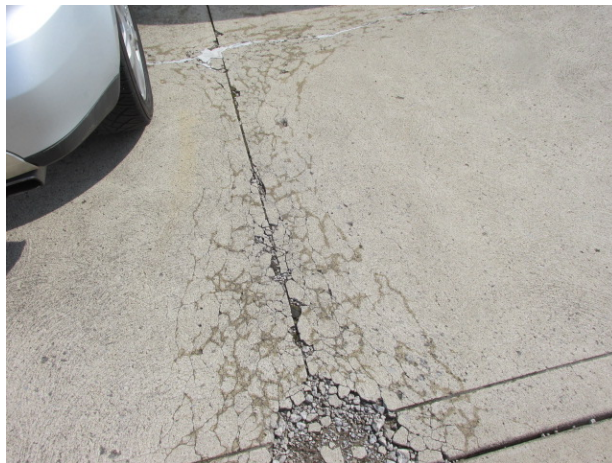
Cracks and deterioration at driveway
